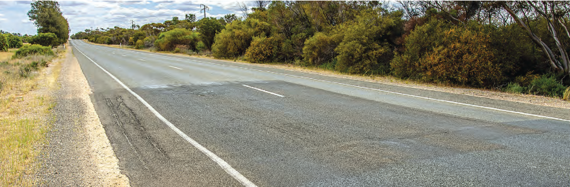
The section of Ramco Road that is causing concern to motorists. PHOTO: Paul McCormick
