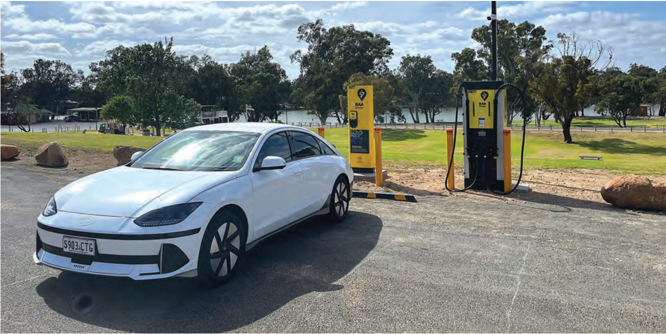
The rapid 150kW charger that was recently installed at Morgan. PHOTO: supplied
