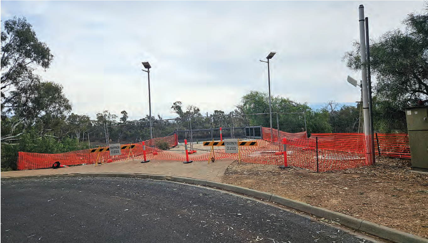
The stairway that connects William Street and the Loxton river front has only recently been assessed following damage during the 2022-23 flood. PHOTO: Stephanie Thompson
