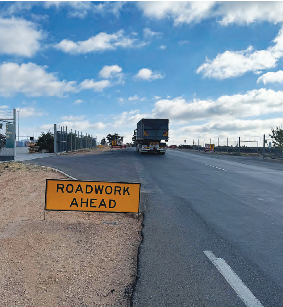
After repeatedly repairing a section of Hoskin Road, in Berri, the local council has decided to upgrade the surface from bitumen to concrete. PHOTO: Paul Mitchell
