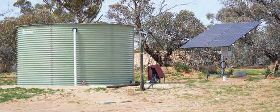
The new water tank with solar underwater pump.
